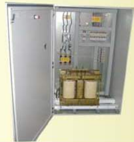
Power Distribution Panel
