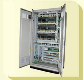
Wired PLC Panel
