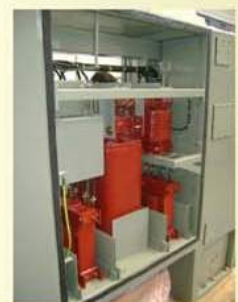
AC Loco Panel
